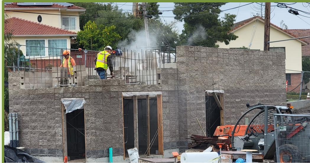
Trash and Generator Enclosure
