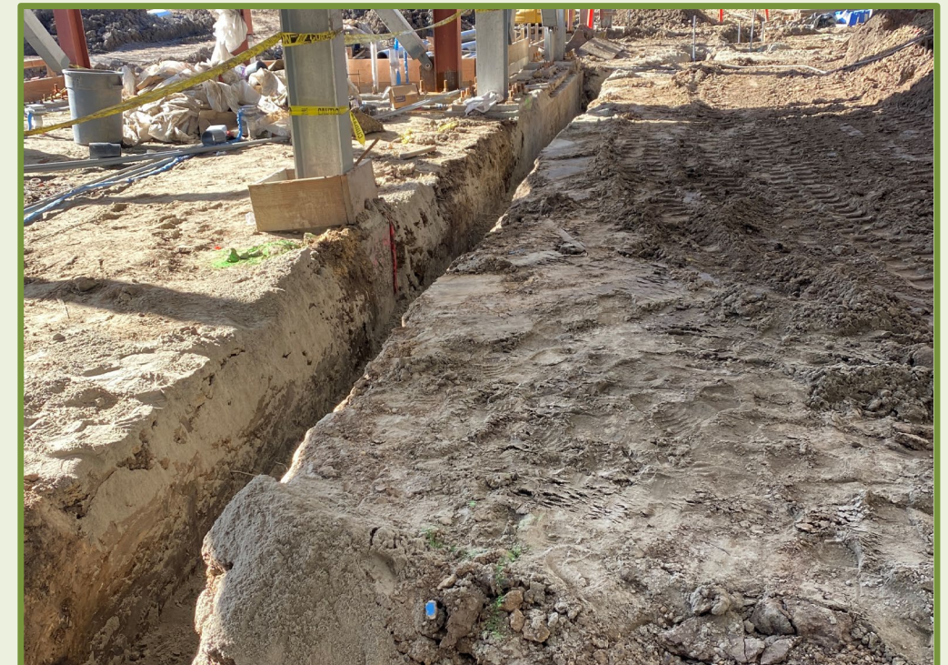
INDOOR POOL PLUMBING
