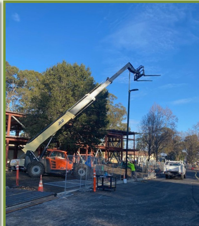
CITY PARK WAY TEMPORARY LIGHT AT INSTALLATION
