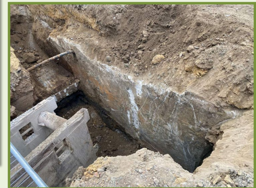
OBSTRUCTION AT SSMH4
