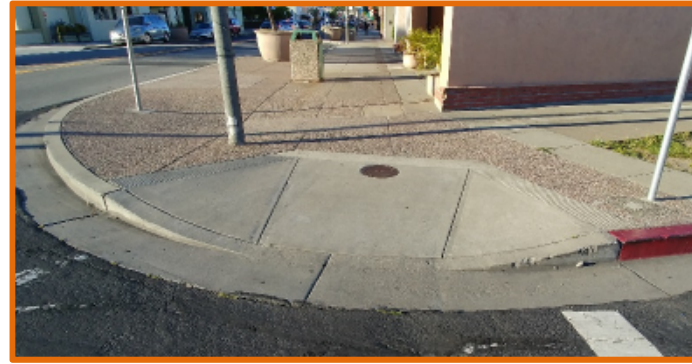
Existing Ramp without Detectable Warning
