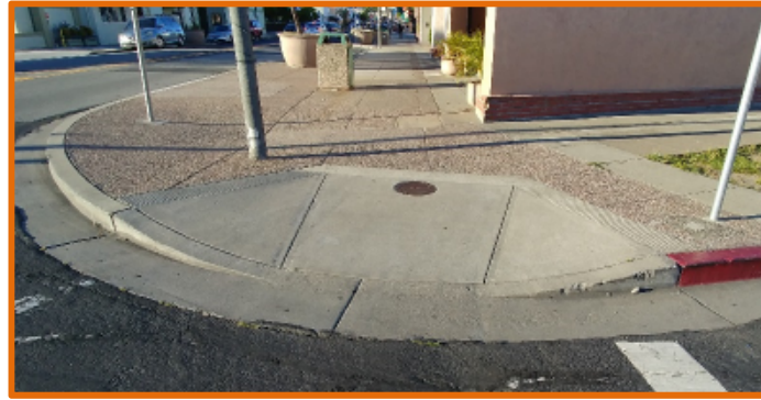
Existing Ramp without Detectable Warning
